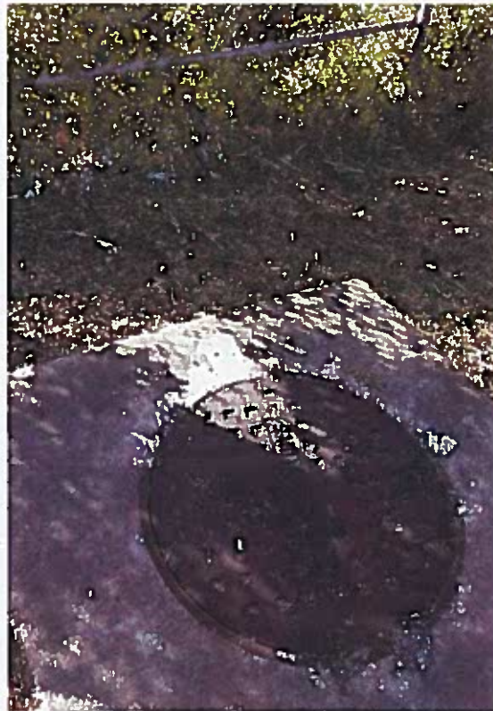
Photo #1 – Sanitary manhole adjacent to Dungca's stream and Guam Waterworks Authority Bayside Pump Station showing visual evidence of overflow into the stream.
